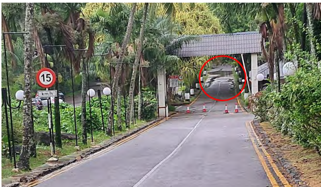
P6 – Water ponding on access road to Berjaya due to lack of drainage as stated in Plate 9
