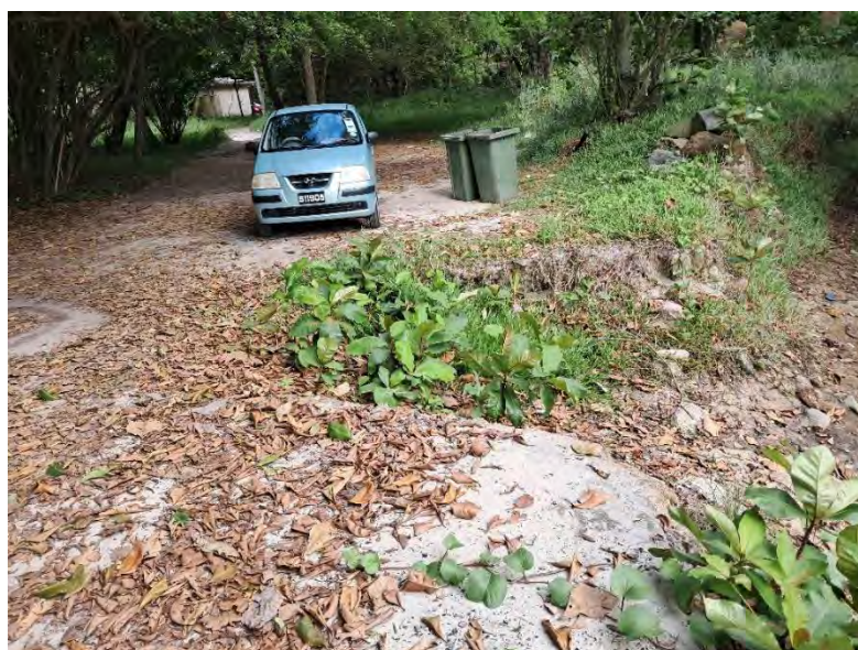
Plate 7 – Channel Bank Erosion and Degradation
